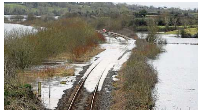
Ballycar, in Clare, pictured in 2014, has been affected by 'significant flood events' in recent years, according to Irish Rail PRESS 22
