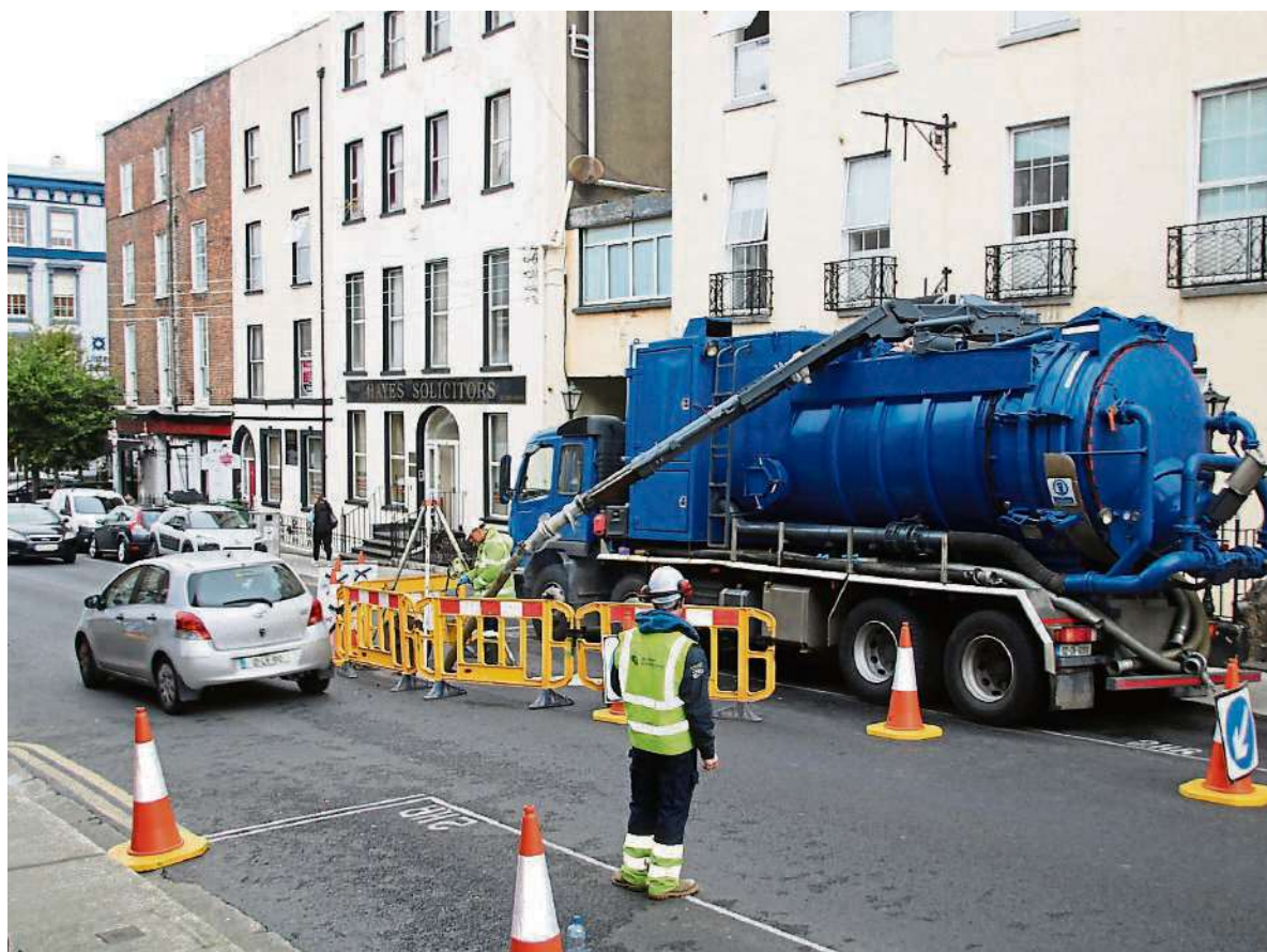
The sewer cleaning works taking place in Glentworth Street this week PICTURE: ADRIAN BUTLER
