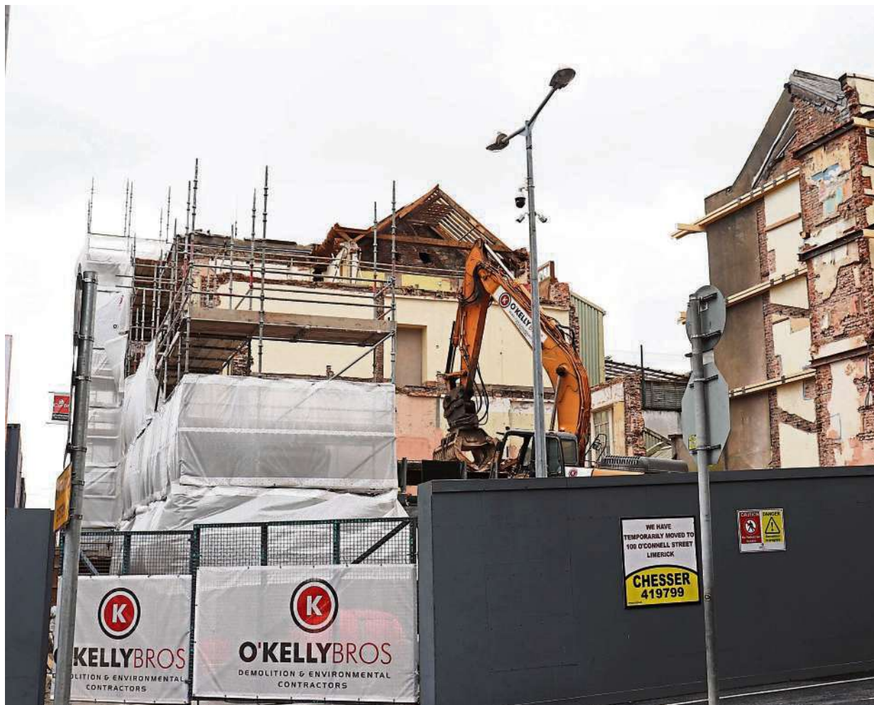
Work on clearing the site for the International Rugby Experience on O'Connell Street is expected to be completed in the next 10 days PICTURE: MICHAEL COWHEY
