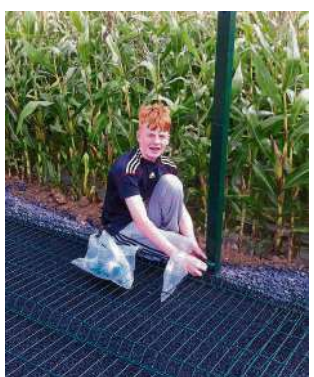
Michael Quinlan placing base hinges in position as the Rosegreen Community Development Plan 2016 - 2020 gathers pace.
